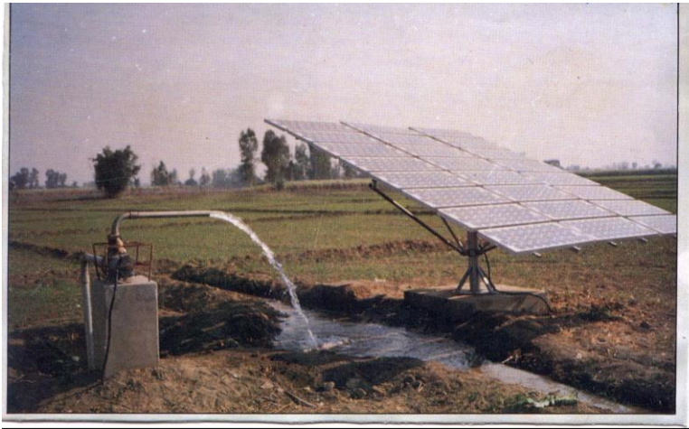
Fig :2. Solar water pumping system
